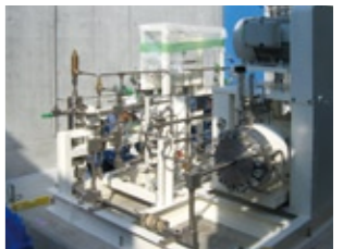
Hydrogen condensing machine
