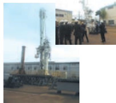
Operational test for a loading arm with an ERS installed
