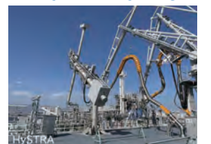
Steel tube loading arm for liquefied hydrogen Developed in collaboration with Kawasaki Heavy Industries, Ltd. Photo courtesy of Kobe Hydrogen Base (Hy touch Kobe/HySTRA)
