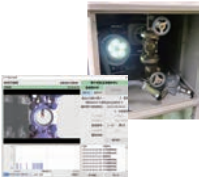
Odor addition equipment, Odor addition monitoring system (dashboard sample)
